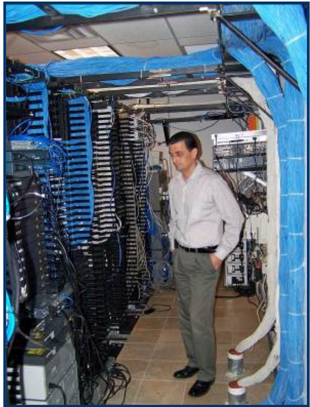
Eddie Mustafa, Systems Manager, shows off the professional level of installation and cabling FFP has accomplished in their Computer Center
